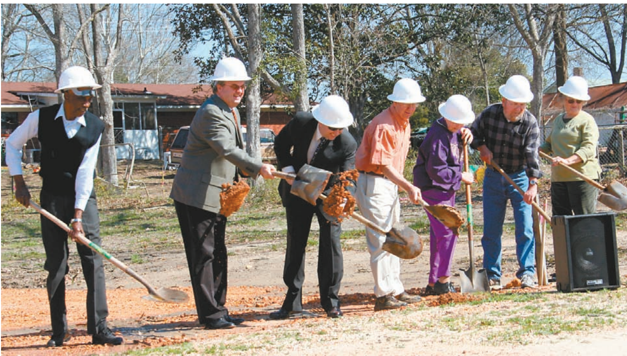
Local officials break ground on a new senior center in Eclectic. The construction of the center was made possible with CDBG funding.
